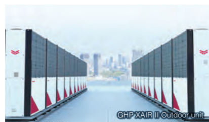
GHP Technology Promoting Energy Conservation
